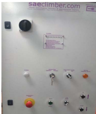
Diagnostic alarm lamps on board
